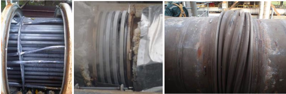
Figure 17: Buckled tubes, corroded expansion joint and “squirmed” expansion joint [2]
