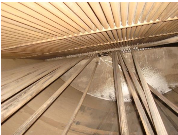
Figure 11: Impingement rod damage as inspected [2]
